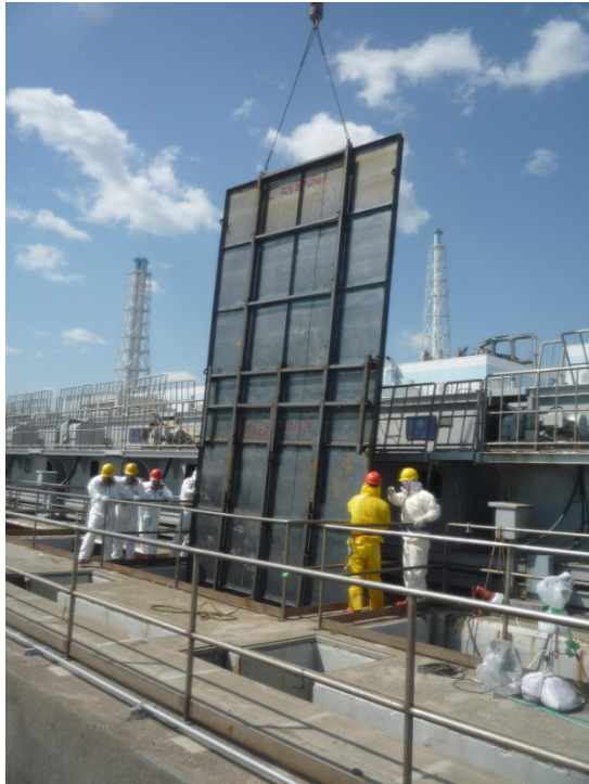
Sluice Gate to Minimize Outflow To Ocean
