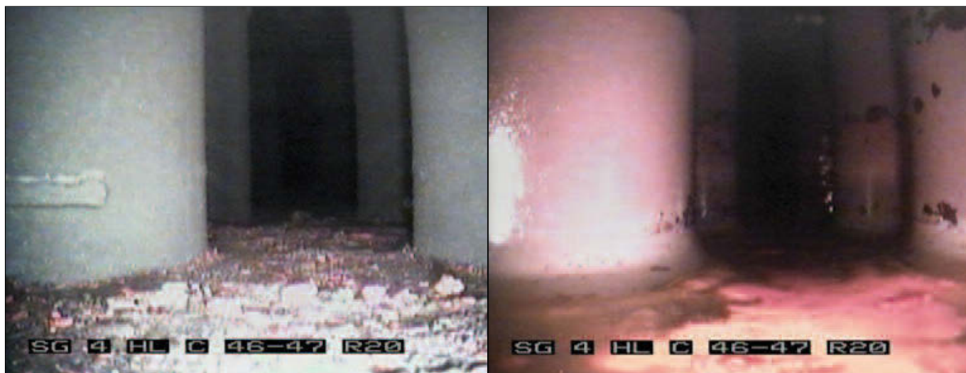
Comanche Peak-2 steam generator 4, Column 46/47, Row 20, pre-sludge lance (left) and post-sludge lance (right). The overall process for all the steam generators removed 85 percent of the sludge estimated to be in the TTS area of the steam generators. (Due to schedule considerations, photos were not taken of steam generators 1 and 2.)
