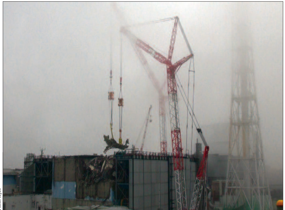
In very foggy conditions on August 2, a crane lifts the severely damaged fuel handling machine (FHM) from the Fukushima Daiichi-3 spent fuel pool.
