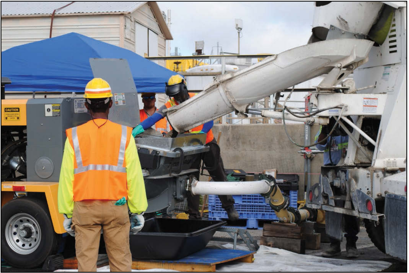
A cement truck begins the initial pouring of grout into Tank 16 at the Savannah River Site on June 2.
