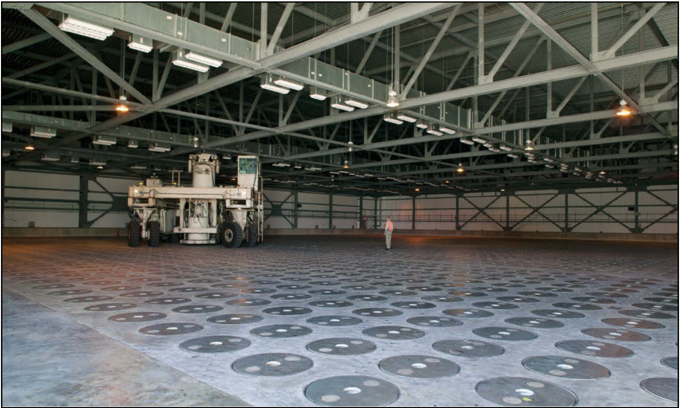
Glass Waste Storage Building 1 at SRS is the interim storage facility for vitrified waste after being treated at the DWPF. The vehicle, called the shielded canister transporter, transports canisters one-by-one from DWPF to the Glass Waste Storage Buildings.
