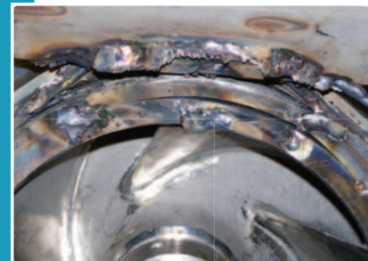
Rotor was damaged due to pump running dry for approximately 30 minutes.
