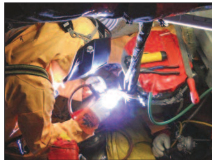
Tri Tool's welders at Sequoyah Nuclear were tested and qualified to TVA's Quality Program and welds performed by them exceeded all acceptable, prescribed standards.
