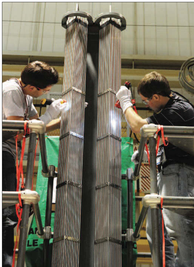
◀ On the refueling floor in Fermi-2's reactor building, two engineers inspect new nuclear fuel, looking for any imperfections.
