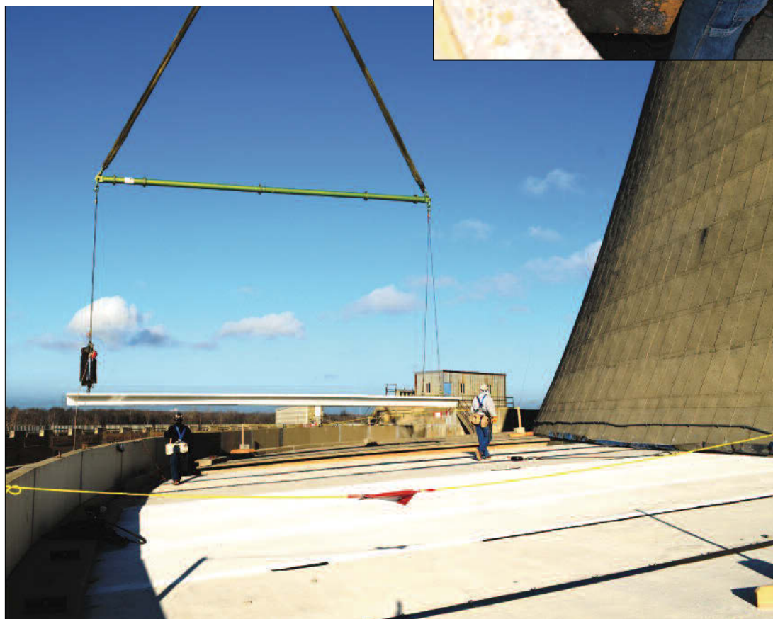
◀ A 160-foot-tall, 240-ton crane was used to replace 10 of the canopy covers on Fermi-2's north cooling tower. Each canopy cover weighs 13 200 lb, is 40 feet long, and measures 8.5 feet wide at one end and 6.5 feet wide at the other end.
