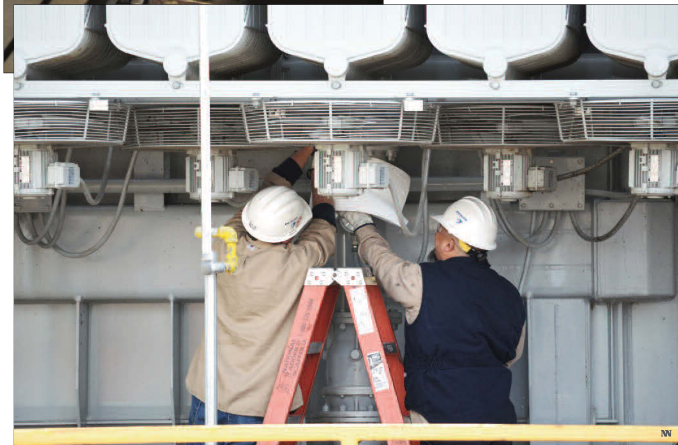
▼ Fermi-2 workers prepare to change out four oil pumps on one of the plant's main unit transformers.
