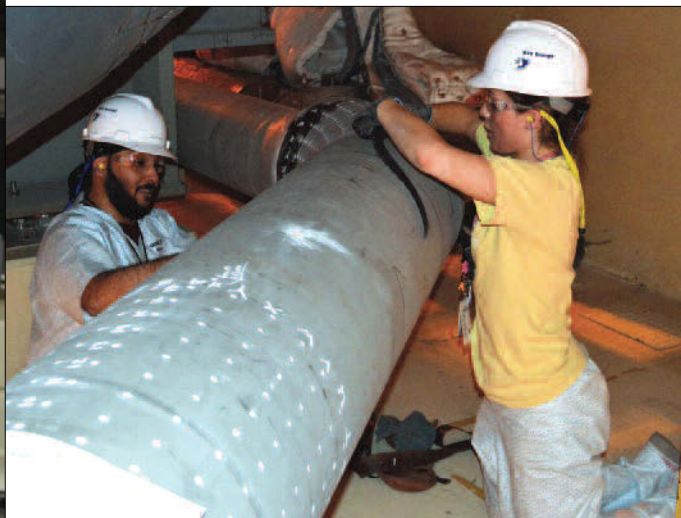
▲ Satbir Singh (left) and Elaine Belenky—both nuclear engineers—work on Fermi-2's flow-accelerated corrosion program. Pipe wall thickness is tested during each outage, and if the pipe walls are found to be thinner than allowable, corrective action is taken.
