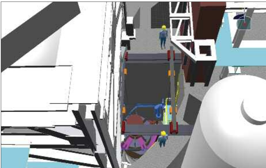
The beam structure between the two figures in yellow hard hats is one of two interferences detected by modeling and simulation during preparations to remove the RCP motor.
