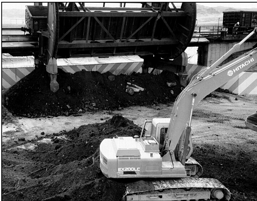
Work at Envirocare of Utah's low-level waste disposal site. The company has applied for a license amendment to allow it to take Classes B and C waste.
