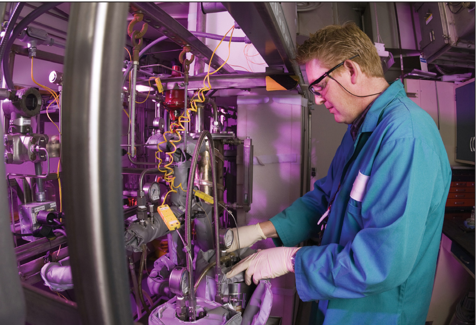
Howard Clemetson, with Areva, installs the removable insulation on the extractor vessels in preparation for starting up the pilot plant.
