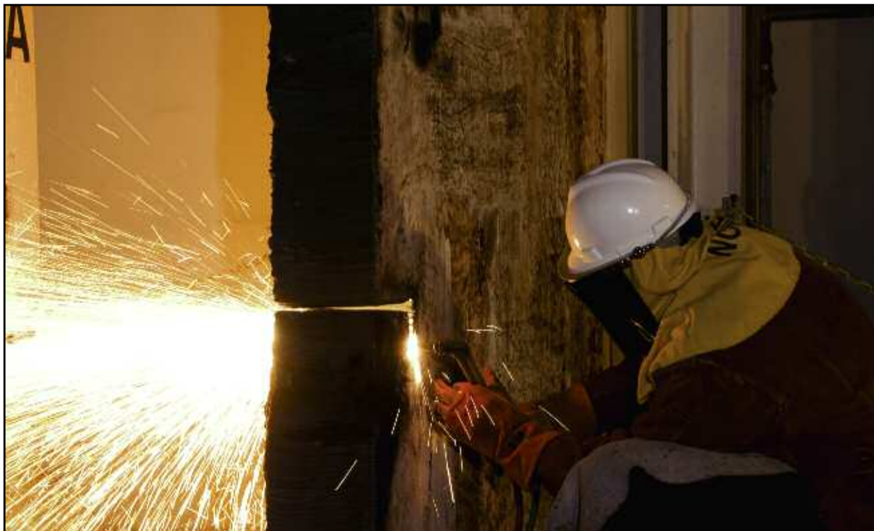
Phil Carter cuts through one of two 8-inch-thick carbon steel doors that shielded reactor workers from the reactor during operation. The door was cut to gain access to equipment that had to be removed.
