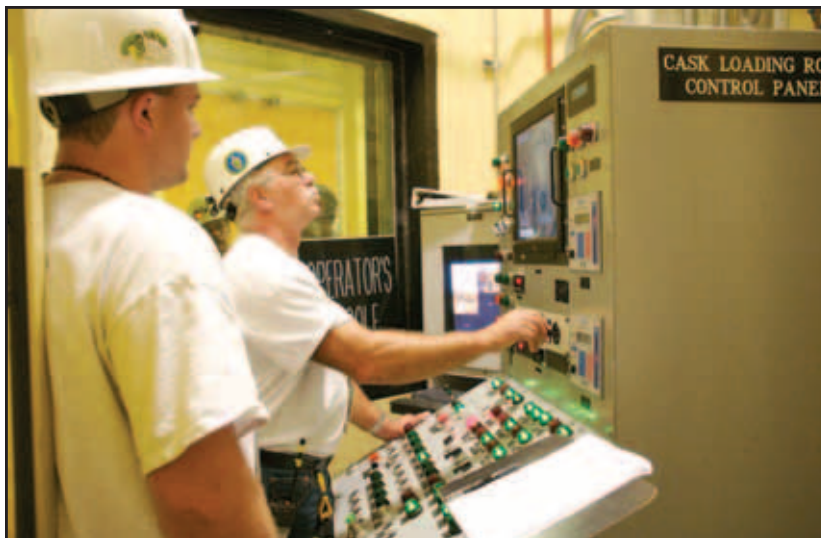
In a simulation exercise, workers at the control panel watch an RH waste cask being loaded into the facility cask, which will then be emplaced into a horizontal borehole in the underground WIPP burial facility.
