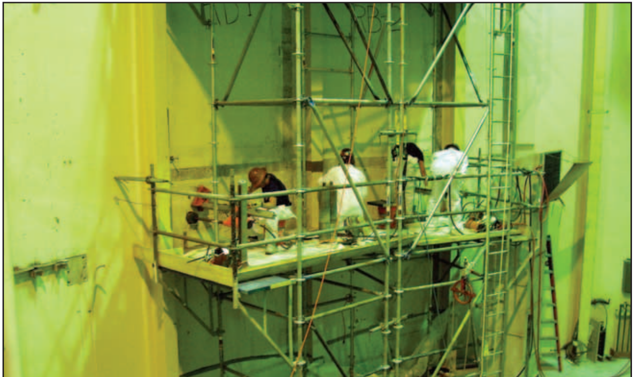
Rigging holes being drilled in the La Crosse reactor building to support vessel removal.
