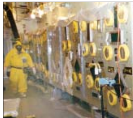
The last glovebox at Rocky Flats being prepared for removal. For more on the winding down of the Rocky Flats clean-up project, see the article beginning on page 39
