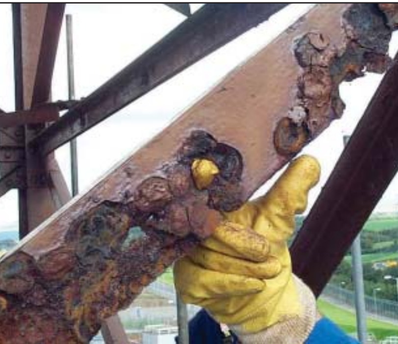
View of structural damage of east tower steelwork prior to the refurbishment necessary to gain access to the tunnel roof.
