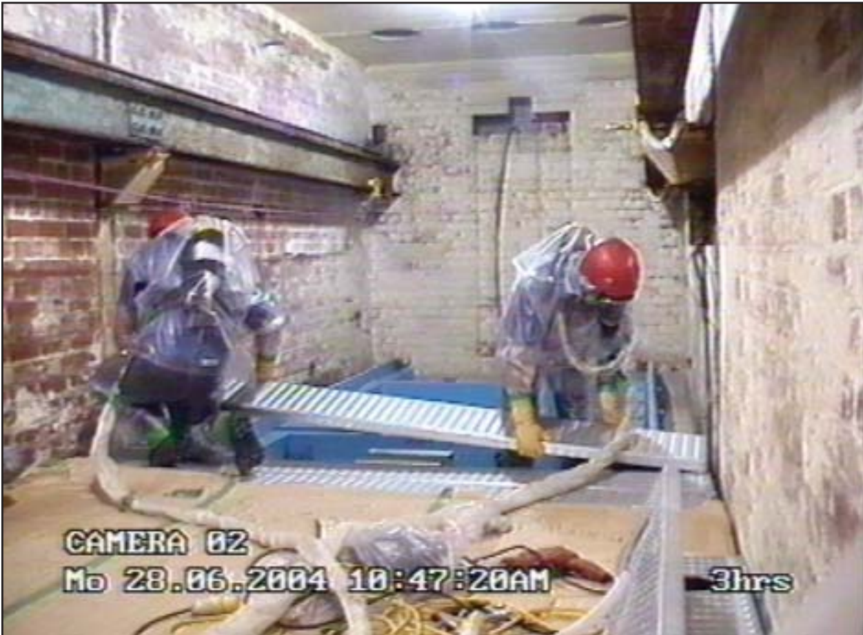
Workers dressed in supplied-air suits install decking material over the waste charge holes. (Photo taken from a video.)
