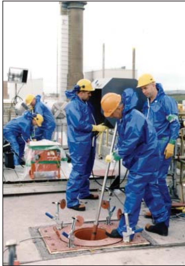
Working on top of the 20.85-m facility, workers dressed in protective gear use a Pokey Stick, designed by the group, to push waste located in the tunnel down into the charge holes that lead to the waste silo.
