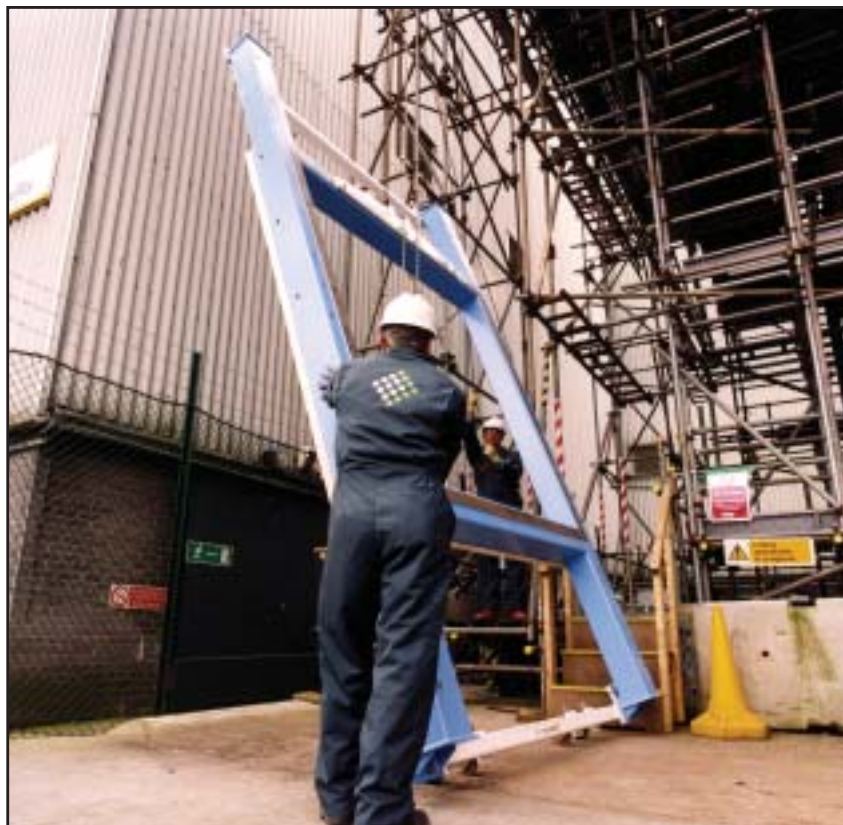
Workers hoist an h-frame mount used to cover the charge holes in the tunnel of the Pile Fuel Cladding Silo. These frames provided workers with a stable base to install decking and the waste charge hole covers.
