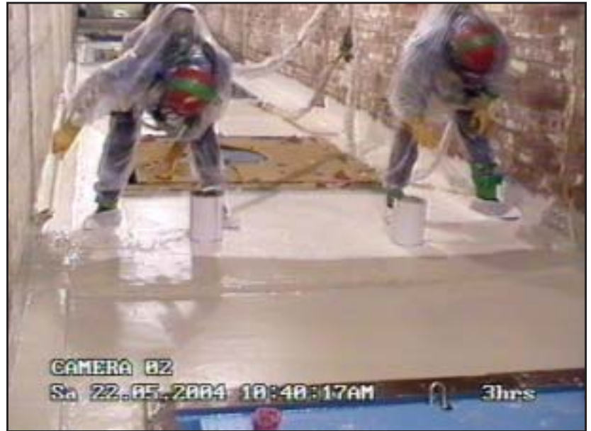
Preparing the tunnel for demolition, workers dressed in supplied-air suits apply the final coat of paint, sealing the waste charge holes off from the tunnel. (Photo taken from a video.)
