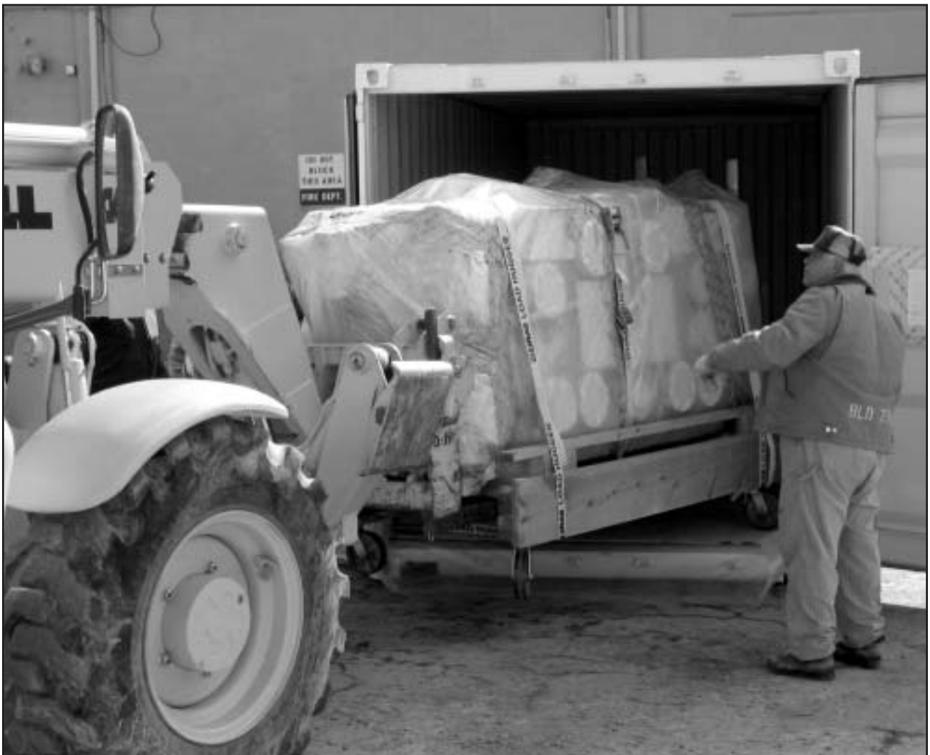
Building 771 workers at the RFETS move a glovebox into a waste crate in preparation for transport to disposal at the Nevada Test Site.
