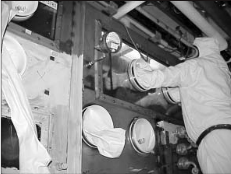
A worker in Building 771 applies decontamination solution to the inside of a glovebox.
