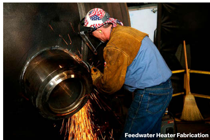
Feedwater Heater Fabrication
