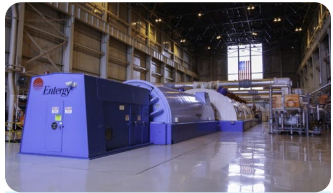
Indian Point-3's turbine hall and generator. (Photo: Entergy)
