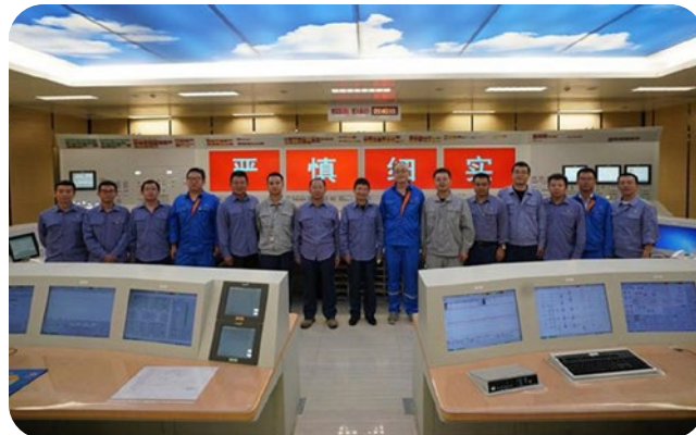
Workers in the control room of the Honghanye-5 reactor. (Photo: Liaoning Hongyanhe Nuclear Power Company)
