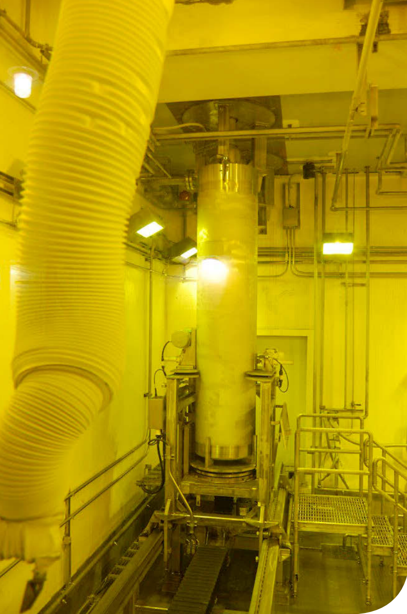
A cell within the IWTU where canisters are filled with solidified waste.
