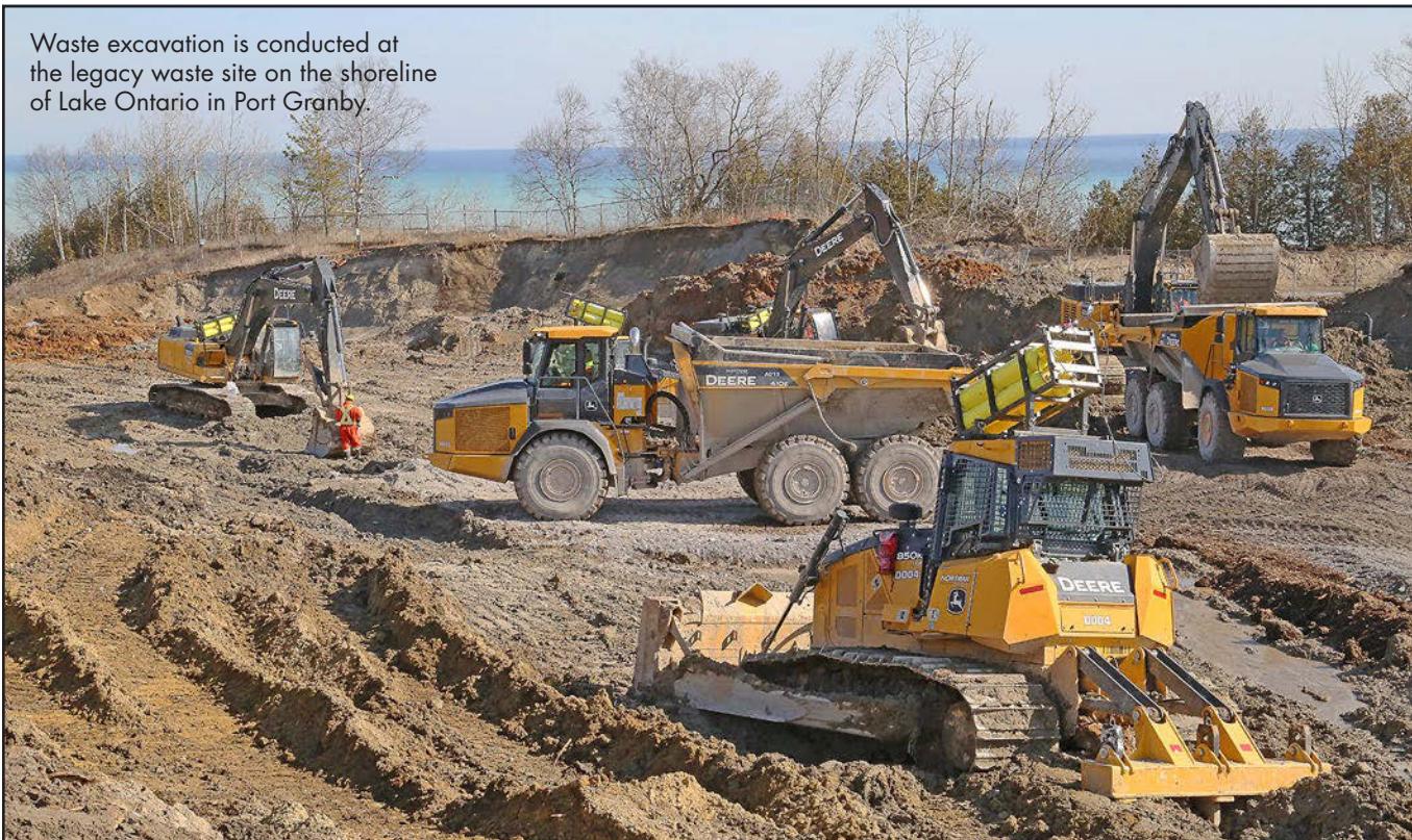
Located at the site's long-term waste management facility, the Port Granby Project wastewater treatment plant uses a two-stage process—biological treatment and reverse osmosis—to remove a wide variety of contaminants from the wastewater. All solids removed through the process are bagged and deposited in the engineered storage facility on-site.
