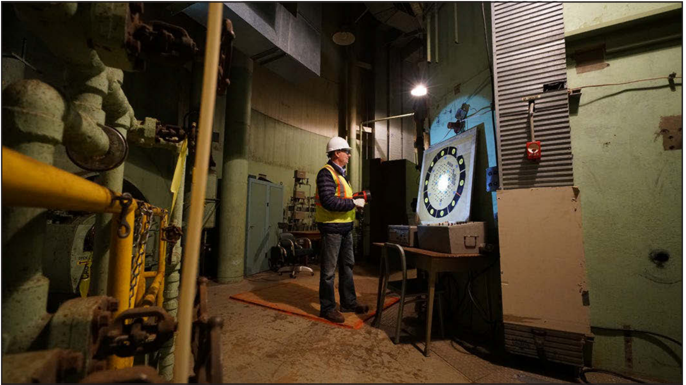
In 2009, UA received funding from the Department of Energy to perform site characterization, develop a decommissioning cost estimate, and write the decommissioning plan for SEFOR. Contracted by the university, EnergySolutions completed the work in 2011. SEFOR D&D Project Manager Dean Wheeler, seen here, inspects the facility before deconstruction work begins.
