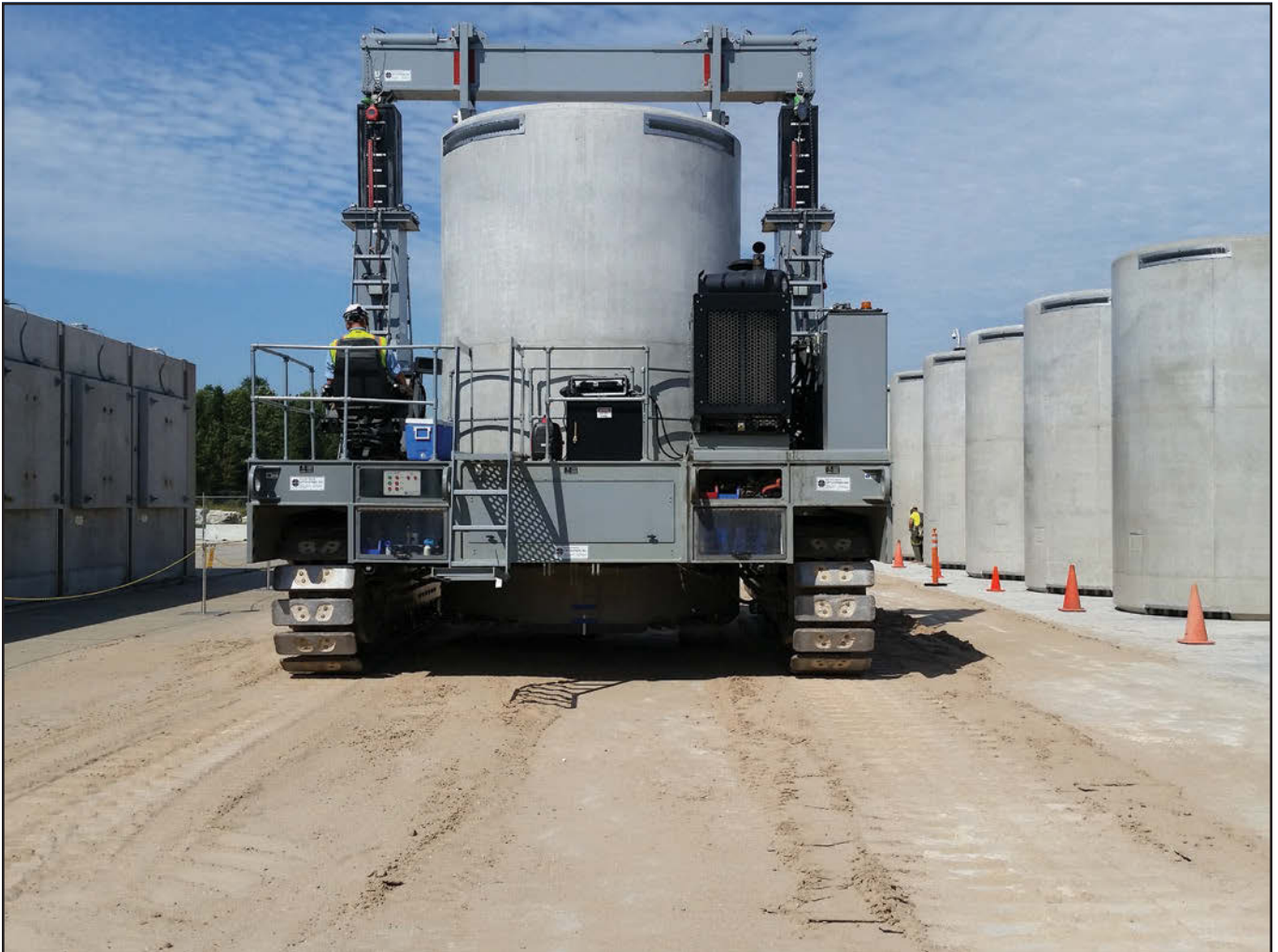
A SNF overpack is moved onto an ISFSI pad. While a national repository has been delayed, the DOE continues to plan for the eventual removal of spent fuel from U.S. power plants. (Photo: NAC International)
