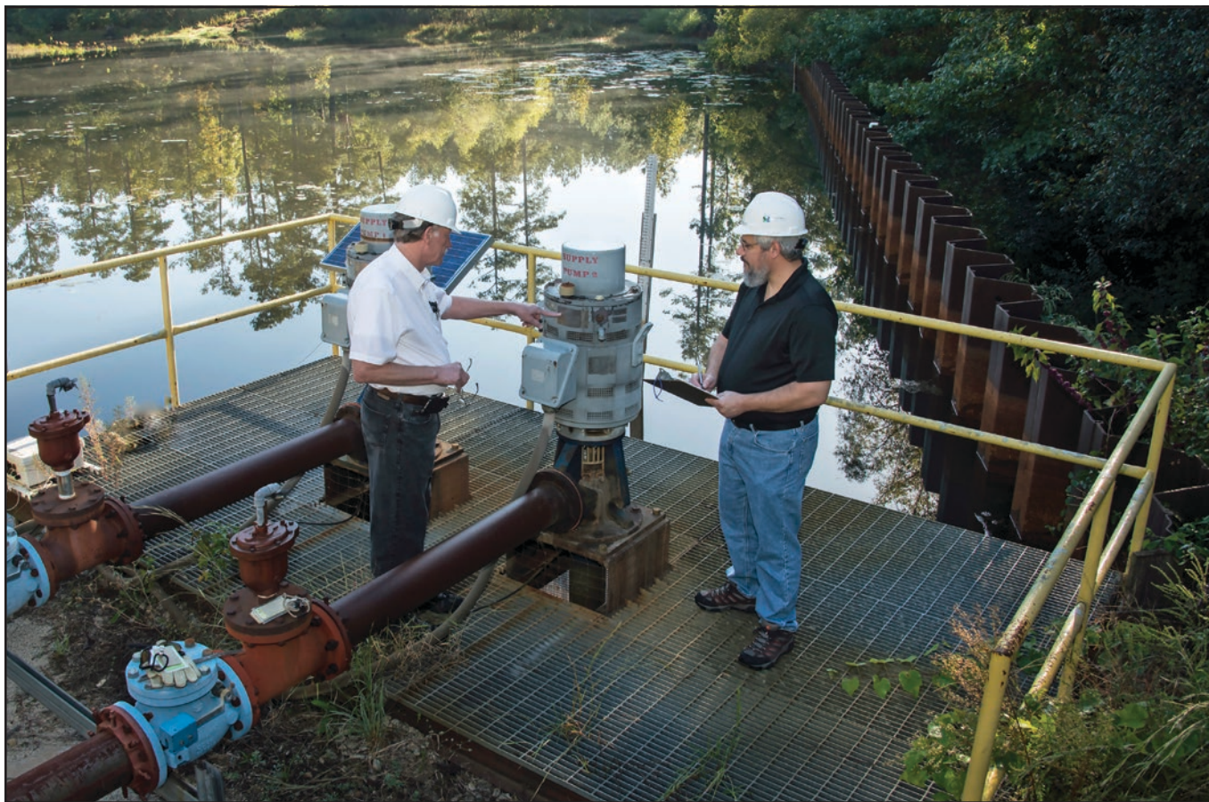
SRNS engineers George Blount and Jeff Thibault inspect equipment that is used as part of an innovative process to remove low-level contamination from groundwater contained near the center of the Savannah River Site in Aiken, S.C.
