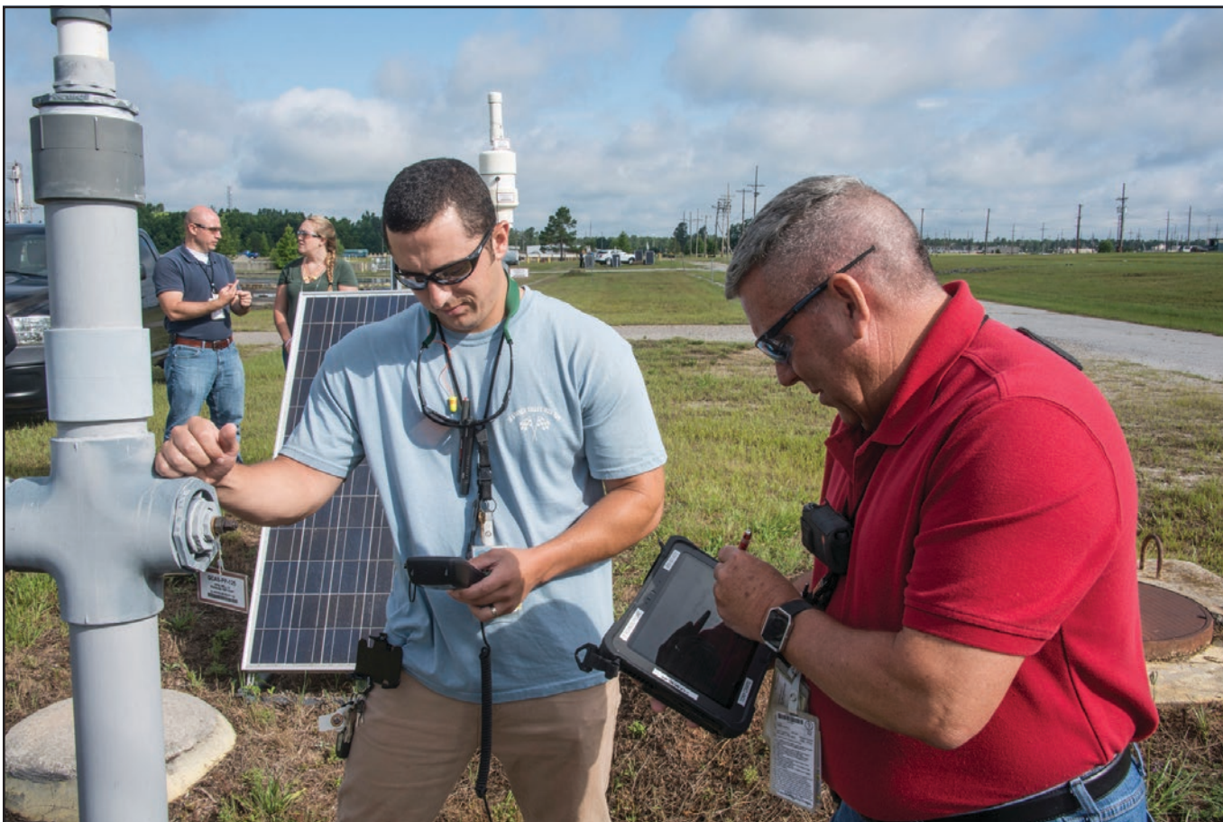
SRNS remote operators Matthew Easley (left) and Tony Craps take readings from a microblower that is used to remove underground chemical solvents. In the background, SRNS Senior Scientist Branden Kramer explains the solar-powered system to intern Sydney Goodlove. (Photos: DOE)
